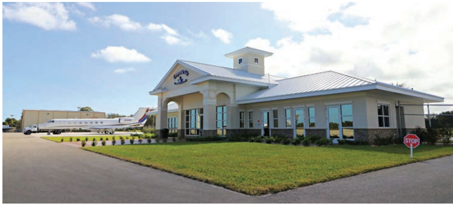
Corporate Air is building a U.S. Customs facility next to the FBO's terminal, allowing Florida's Vero Beach Regional Airport to welcome direct international flights.
