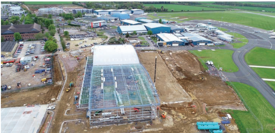
A new 6,000-sq-m hangar under construction at the UK's London Oxford Airport will add much-needed large business aircraft shelter to the airport and the London-area in general.
